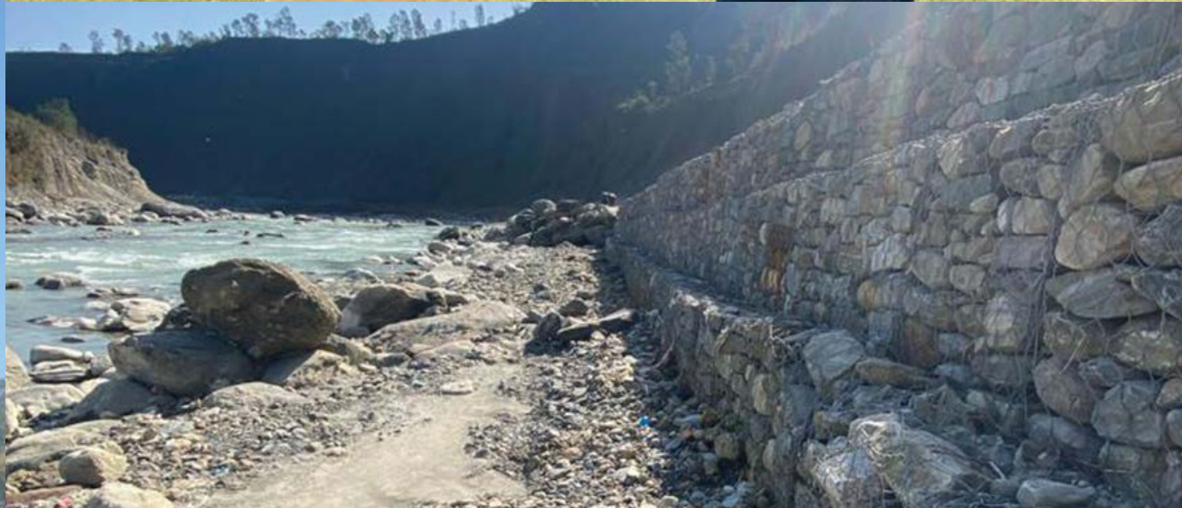
Clockwise from bottom left: Steve Raymond, Give Freedom International CEO, Shudhir, John Sanday Associates (JSA) CEO, and a local community member standing on new retaining wall; Completed riverworks; Rajendra and Samip Shrestha from SMT Building; Completed riverworks retaining wall.
